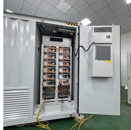
Solar Lithium Battery Pack LBB Series (Horizontal type, 1500 ...
