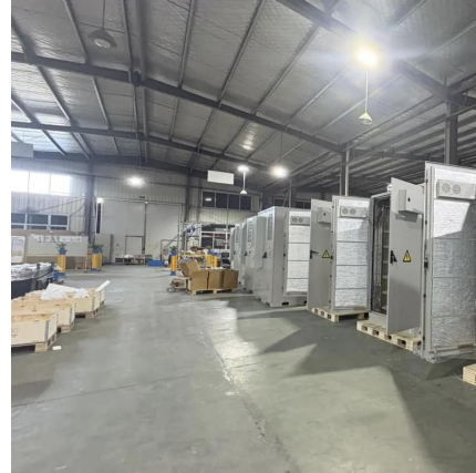
Nicosia photovoltaic power plant energy storage
