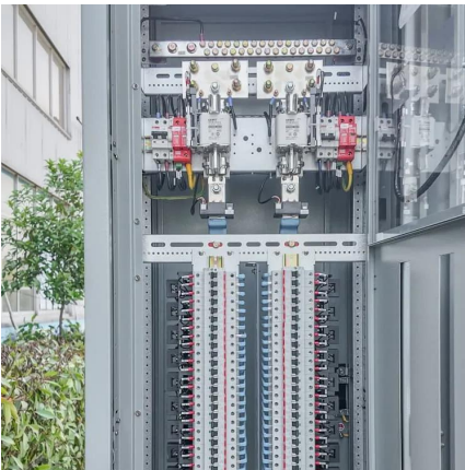
Sunway 1Mw Battery Container Energy Storage System
