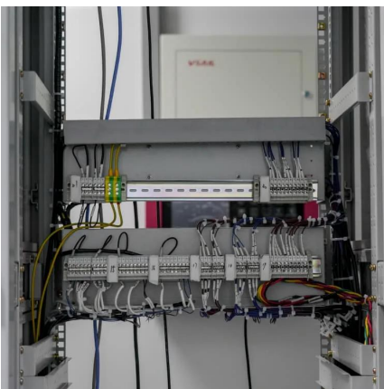
Solar Container Energy Storage System 1mWh Lithium...
