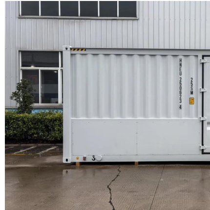
20ft Containe 1MWH Battery Energy Storage System
