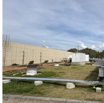
20ft Containe 1MWH Battery Energy Storage ...
