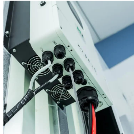
2MWH Containerized Solar Battery Storage ...
