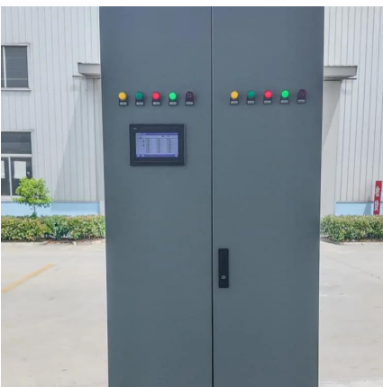
Dawnice Battery , 2MW Energy Storage Container
