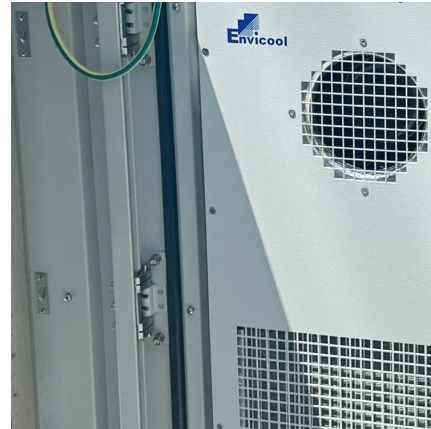
SUNWAY 30KW 51.2KWH Energy Storage System
