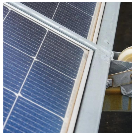
SUNWAY 30KW 51.2KWH Energy Storage System
