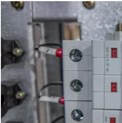
5MWh Container Energy Storage System
