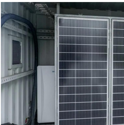
Sunpal Complete Kit Off-Grid Solar Power Energy System
