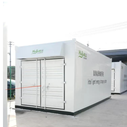
Armenia Photovoltaic Off-Grid Power System
