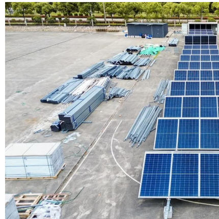
Solar Container , Large Mobile Solar Power ...
