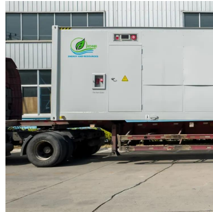
Liquid-cooled battery energy storage system Barbados
