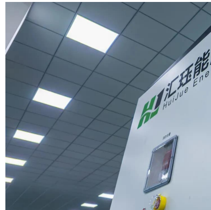
Lithium battery solar container intelligent control system
