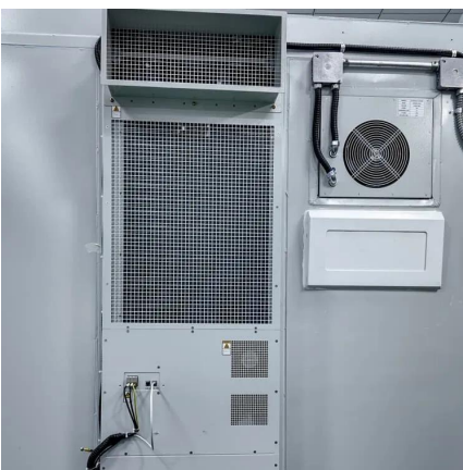
BLOEMFONTEIN BATTERY ENERGY STORAGE COMPANY, Solar
