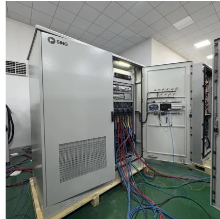
Colombia: 2MWh LFP battery storage unit in ...
