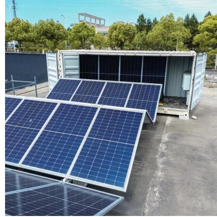
Telecom Base Station PV Power Generation System ...
