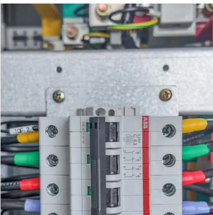
Services - Glass City Community Solar
