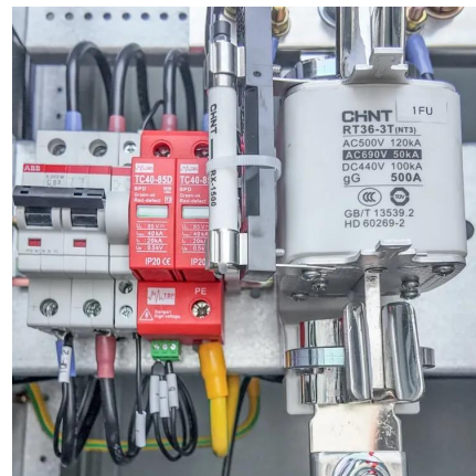
Solar Power Containers
