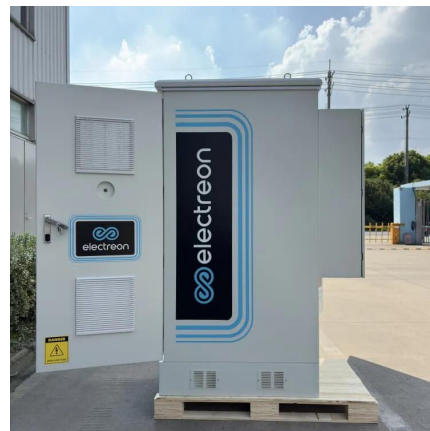
Switchgear Equipment Suppliers, Manufacturer, Distributor, ...
