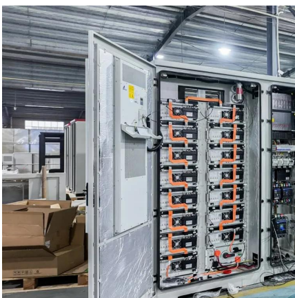
Gabon energy storage photovoltaic power generation ...
