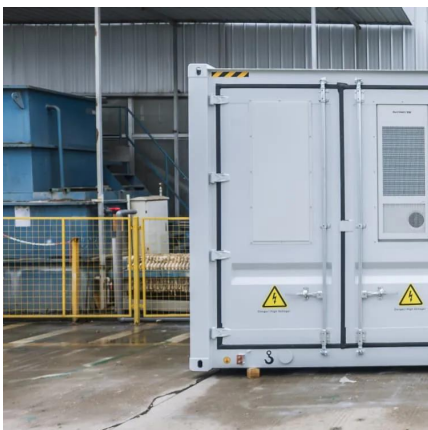
BMS (VRLA) - Narada Power Pakistan
