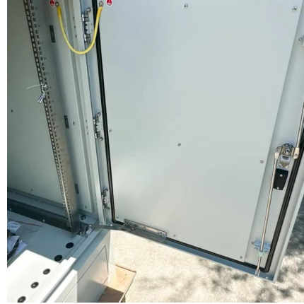
Outdoor Power Panel In Israel
