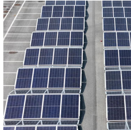
Solarcontainer: The mobile solar system
