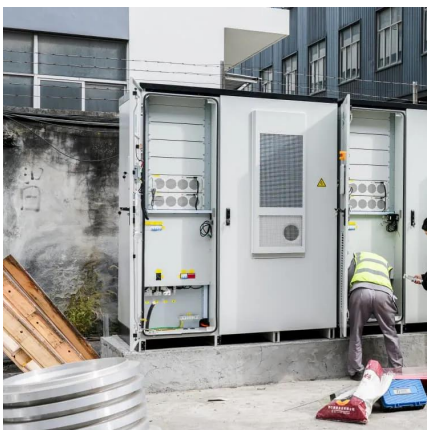
Lithium Battery Energy Storage Cabinet
