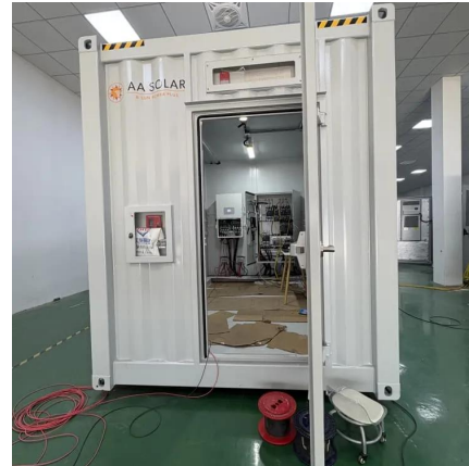
Lithium Battery Energy Storage Cabinet
