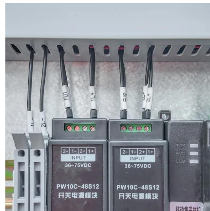
Cabinet Energy Storage System , VREMT
