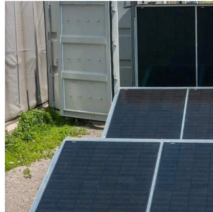
Lithium-Ion Battery Storage Cabinet
