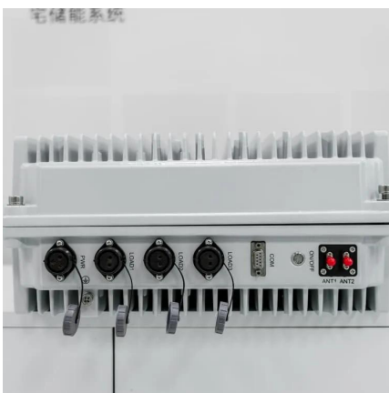
Lithium-Ion Battery Charging Safety Cabinet
