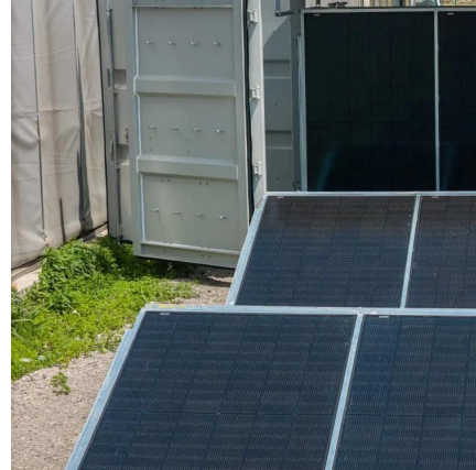
Lithium-Ion Battery Storage Cabinet
