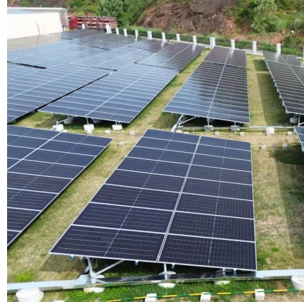
Horn of Africa Solar Panels Plant
