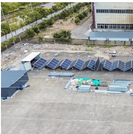
NAURU SOLAR POWER DEVELOPMENT PROJECT - BATTERY ...
