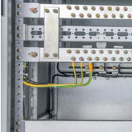
20kW Off Grid solar system (38.4kWh)
