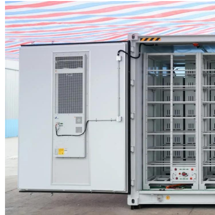
CATL's TENER Stack: 9 MWh Containerized ...
