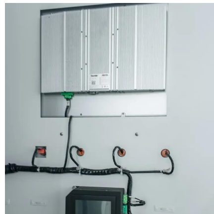
30KW Complete Offgrid Solar Kit
