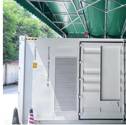
30kW Off Grid solar system (38.4kWh)
