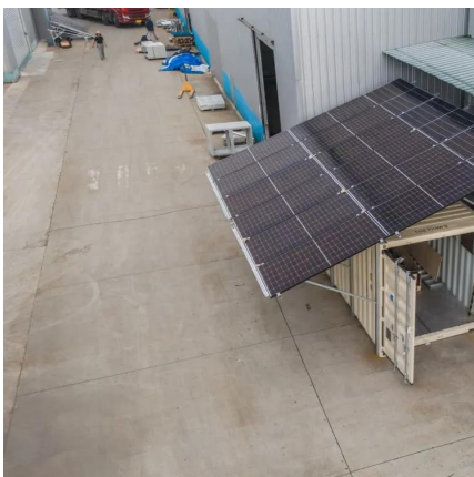
500kw solar system - solar energy storage ...
