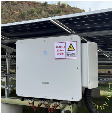
Containerized Photovoltaic Power Plant ...
