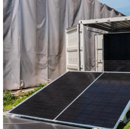
BESS Smart, Battery energy storage systems, Smart ESS, Smart ...
