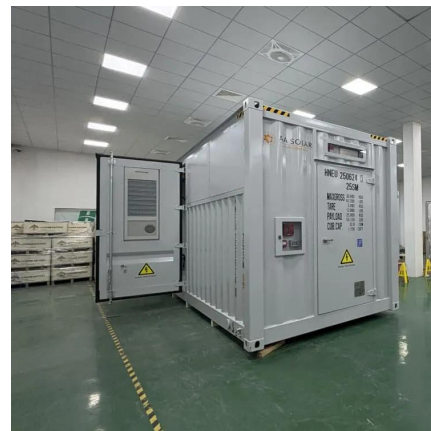
Communication container station energy storage systems
