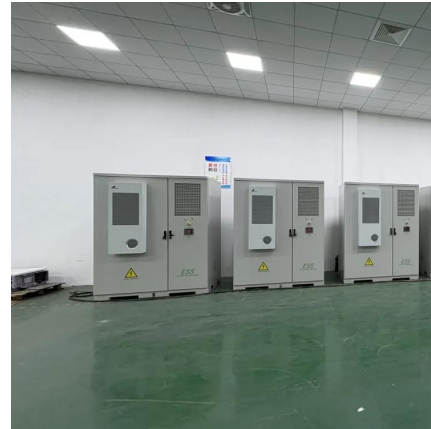
TCOM Solar Communication Tower
