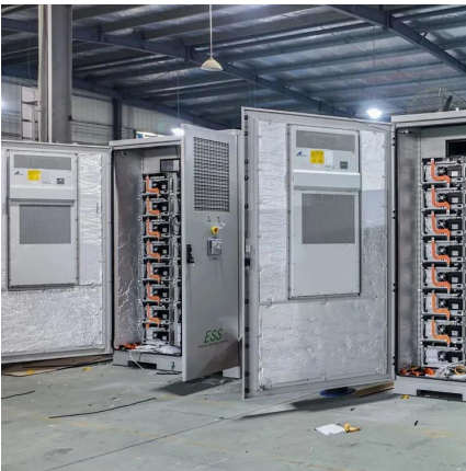
Containerized Energy Storage Systems in El Salvador...
