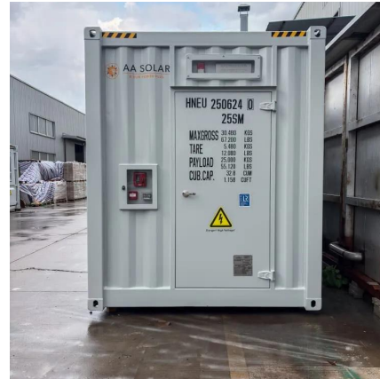
Photovoltaic Energy Storage Container Structure: The ...
