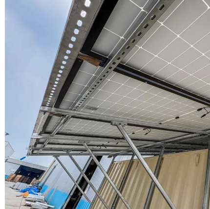
St George Energy Storage Solar Power Generation Project
