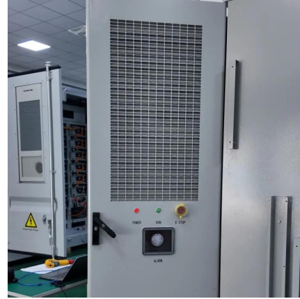
Thailand Electrical Distribution Switchgear ...
