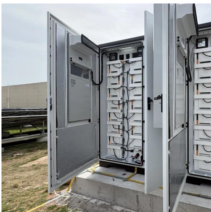
Energy Storage Solution (ESS) , HUAWEI...
