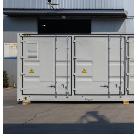
Thimphu container energy storage system
