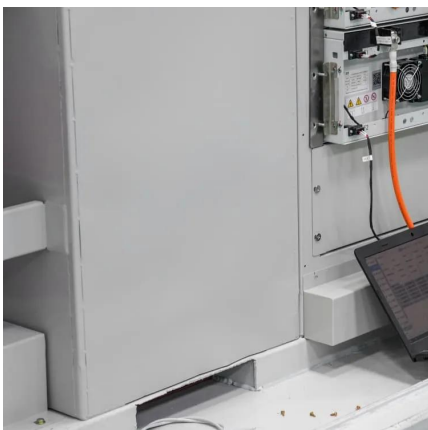
Huawei IDS1000 Container Data Center Solution
