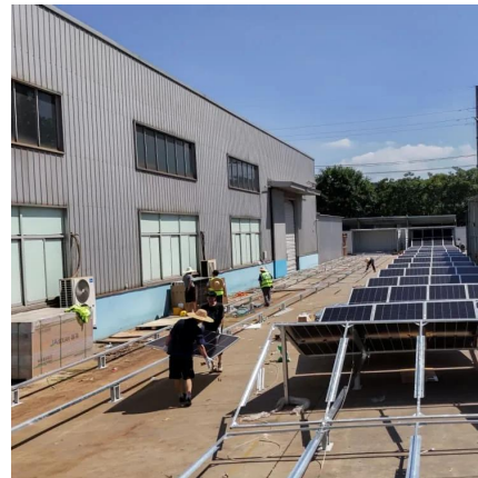
Solarcontainer: The mobile solar system
