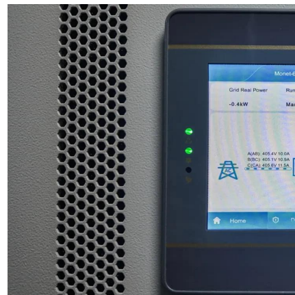
Solar Power for Data Centers and IT Infrastructure
