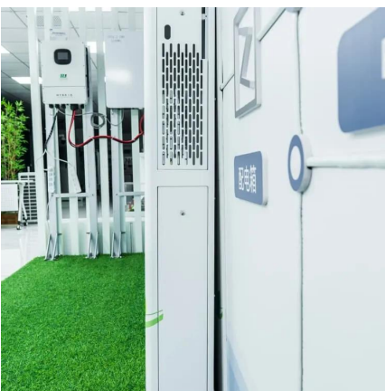
Huawei IDS1000 Container Data Center Solution
