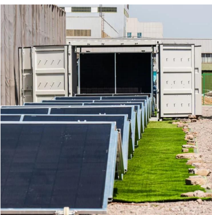
120V 50A Heavy-Duty Energy Storage Battery Cycling Test
