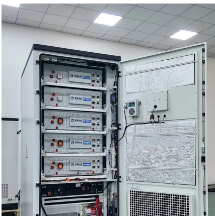
Solar energy and communication battery cabinets
