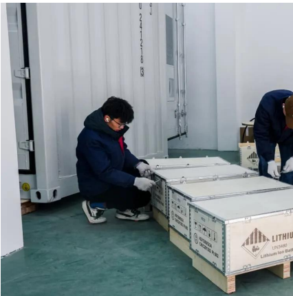
Mobile Solar Container Power Generation...
